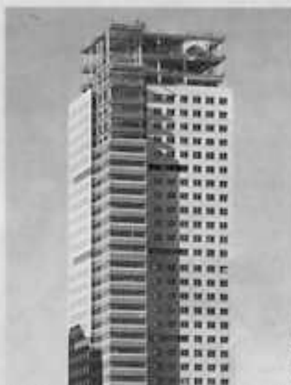
Hartford 21, under construction by Northland Investment, will include a residential tower, retail and office space.
